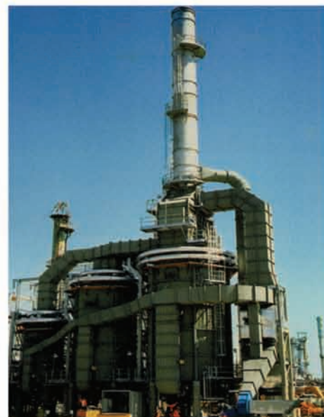
Multi-cell catalytic reformer furnace with combustion air preheat for optimum heat recovery
