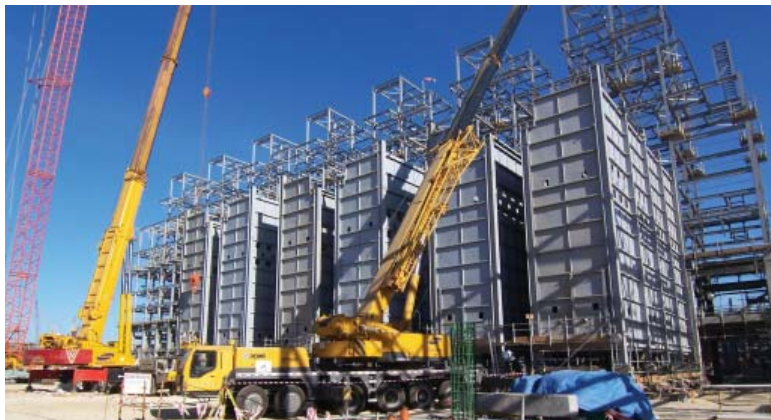
Furnaces supplied on an EPC basis by Selas Fluid
